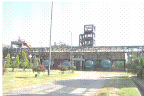
Chlorine Storage Area
