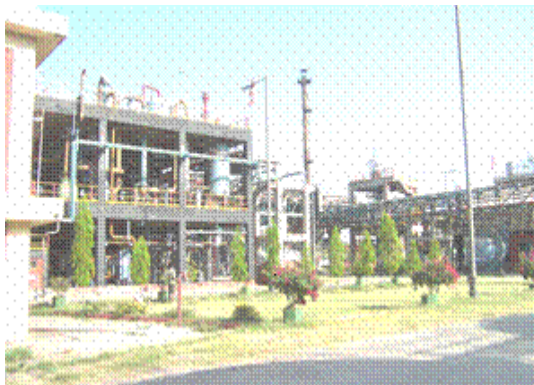
Caustic Soda Concentration Unit & Boiler
